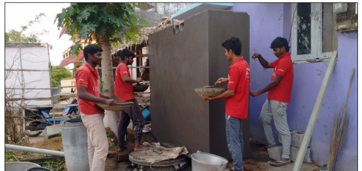
Special Camp of IHHL (Individual House Hold Latrine) construction under the Government schemes of Open Defecation Free (ODF) in Nallambakkam and Nedungundram villages.
